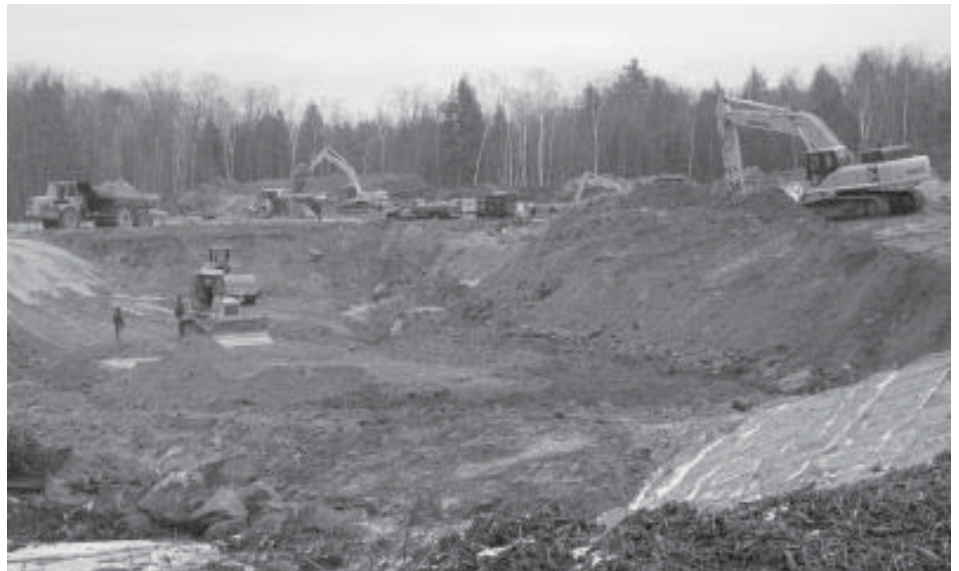
Construction crews work on the Sutton Big Dig preparing the site for new Kearsarge Middle School. Photo by Audrey Sylvester
