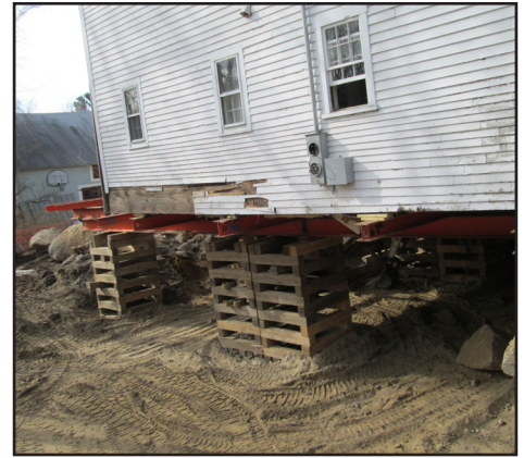
I beams and temporary footings hold the building aloft while a new foundation is poured.
