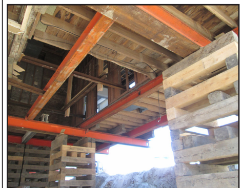
Cribbing under the floor of the building. Old flooring in that area was removed.
