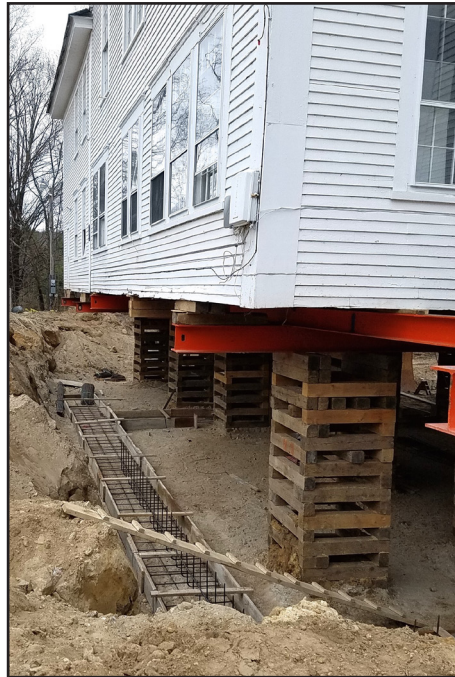
Once the building was raised, work began to lay the footings for the foundation.
