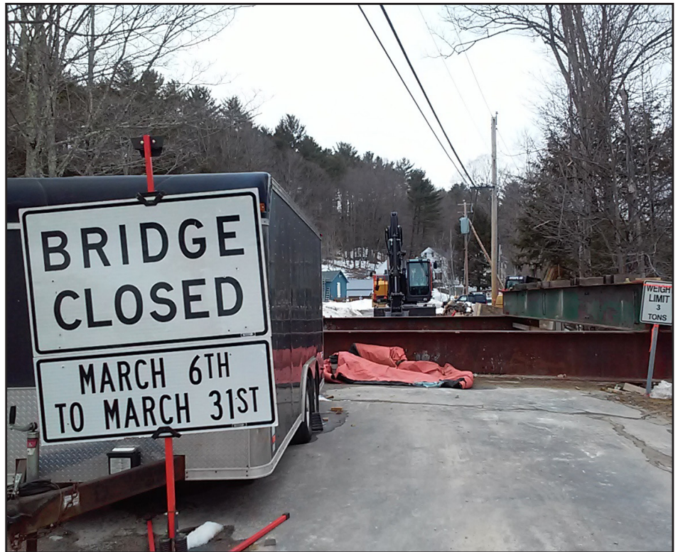
Water Street bridge has been under construction and should be open now.
