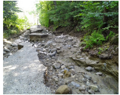
Recent torrential rains did extensive damage to Bradford roads. A large section of Deer Valley Road was washed out. Kudos to Barry Wheeler and his crew for quick repairs.
