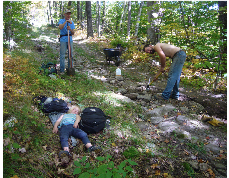
Ed MacLeod, Nathaniel and Emily Bruss all hard at work repairing water bars on Knights Hill Trail.
