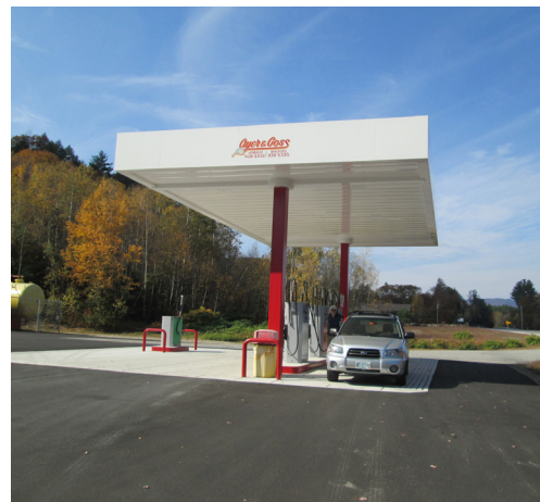
Ayer & Goss erected a new canopy over the pump island on Route 114.
