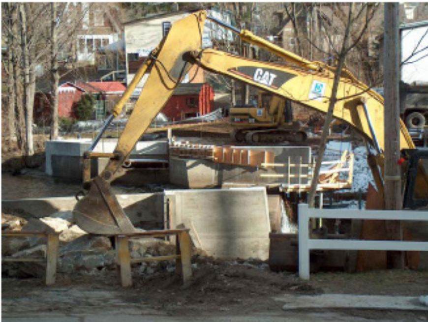
The Lake Todd dam repairs are almost finished. It has passed inspection by a State Dam Bureau engineer and now meets requirements for its "high hazard" class. All that is needed now is some site work, seeding of disturbed areas, paving and a new drain. Come check out the improvements.
