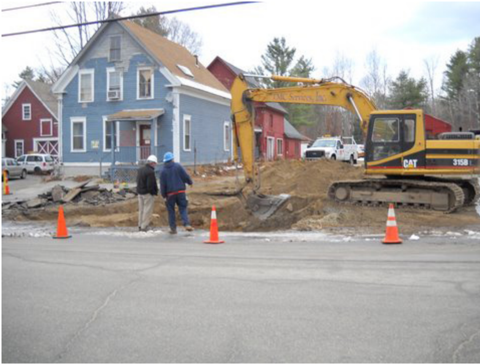
Workers clean up toxic materials from the Ploettner property on Main Street
