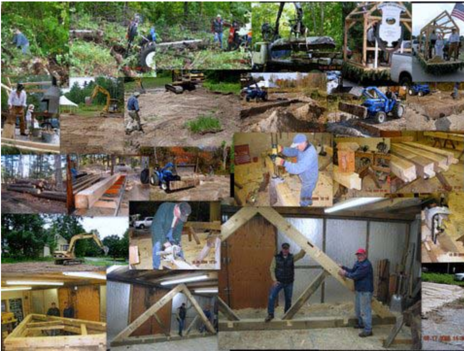
The Blacksmith and Woodworking Shop will be completed in the late spring with a gala raising. The timbers and purlings have been stored inside for the winter.
