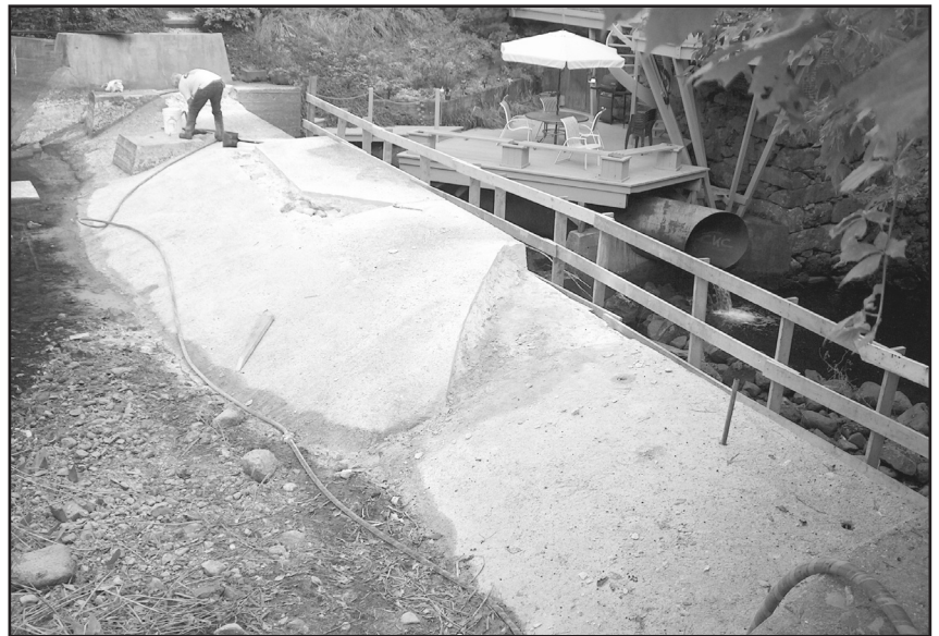
September 23rd: The water is level down and damn repairs begin. The Harris’ deck is high and dry.
