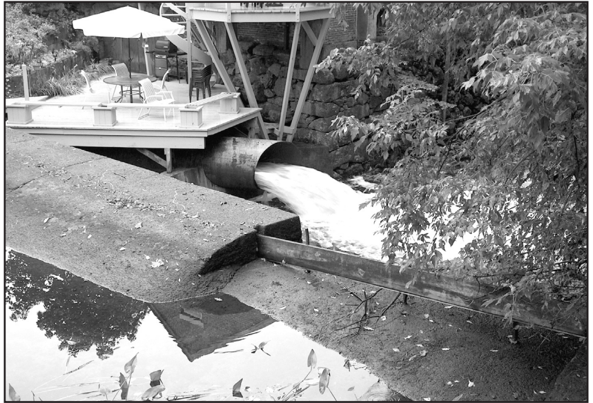
September 16th: Behind the Harris home a view of the damn with normal water flow.
